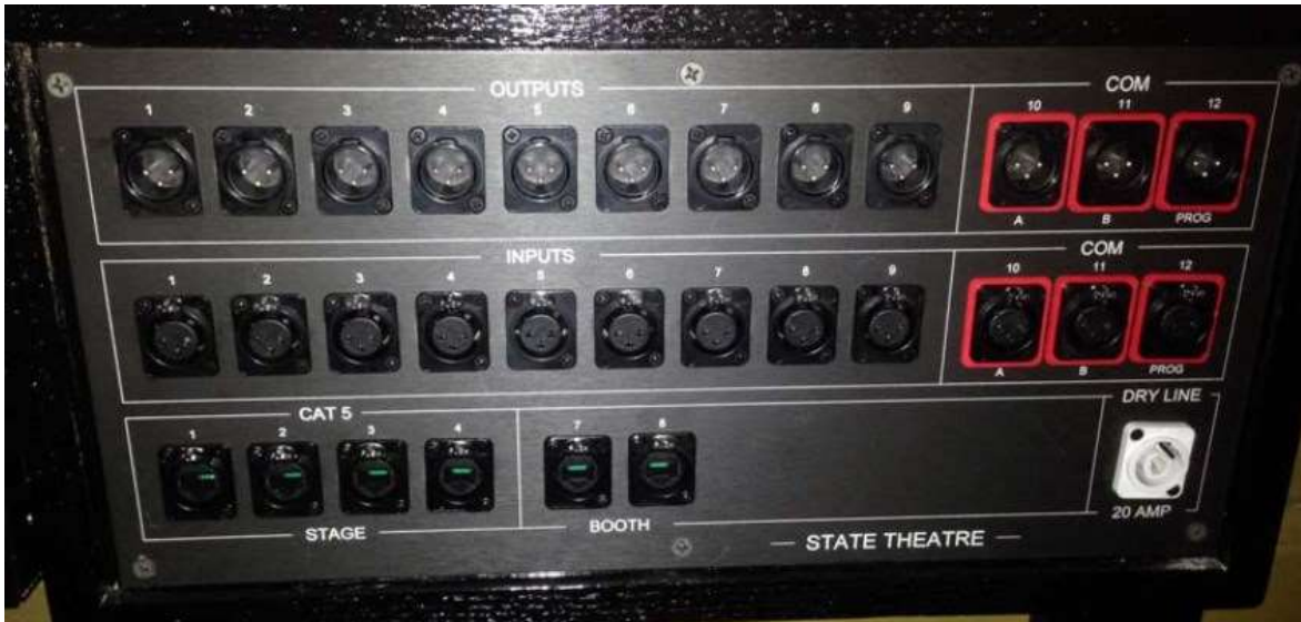
Panel Front of House Center
